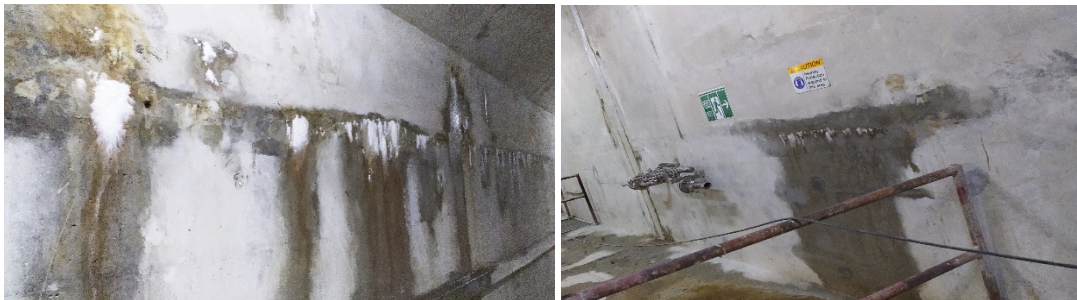
Figure 3: Damp spots and leakage along lift joints at EL1024 and EL1017
