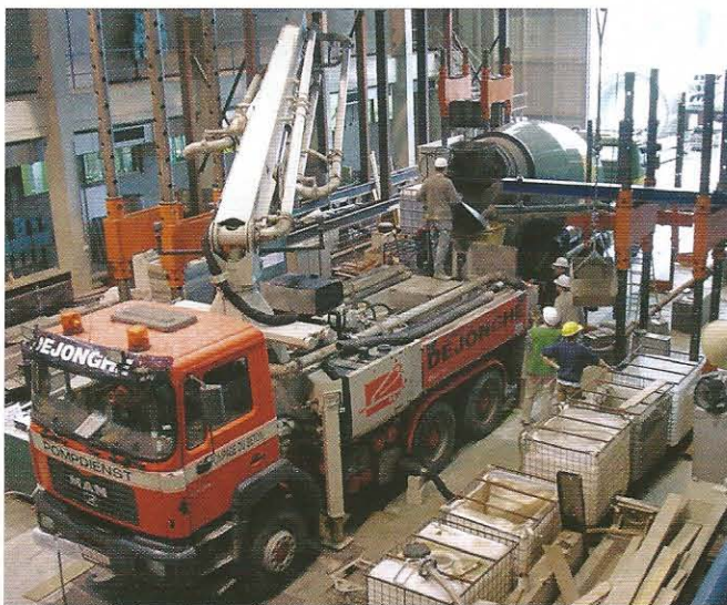
Figure 1. Concrete piston pump.
