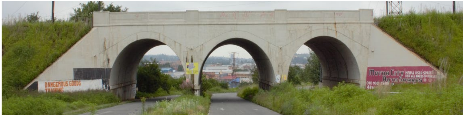
Fig. 3 : North facing view of Railway Bridge on Treu Road and Crown Mines Spur
