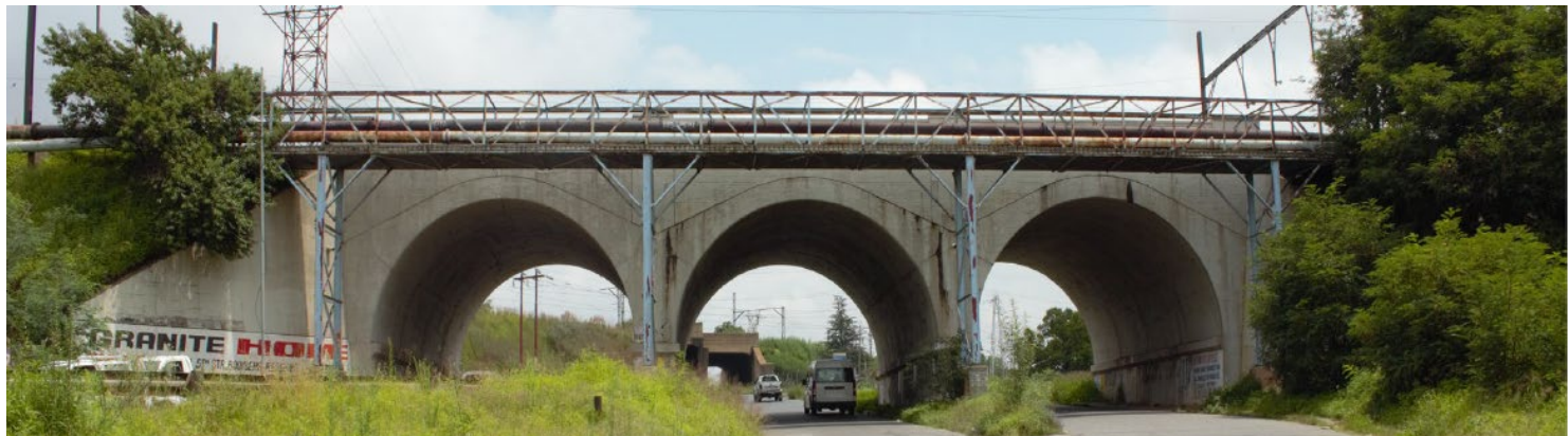
Fig. 4 : South facing view of Railway Bridge on Treu Road and Crown Mines Spur
