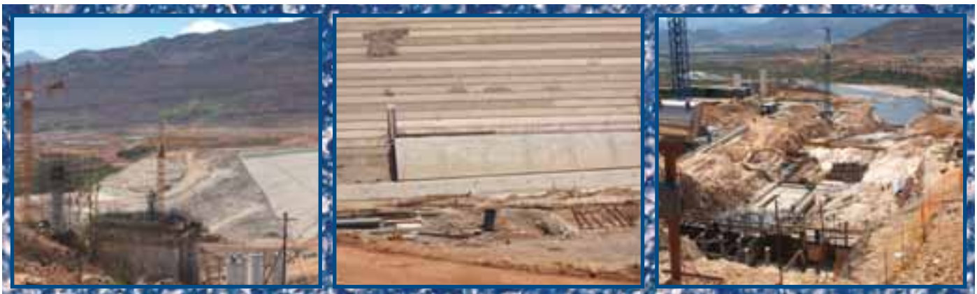
The upstream face of the dam wall, showing earthworks in progress and preparations for the slide-formed concrete face.
