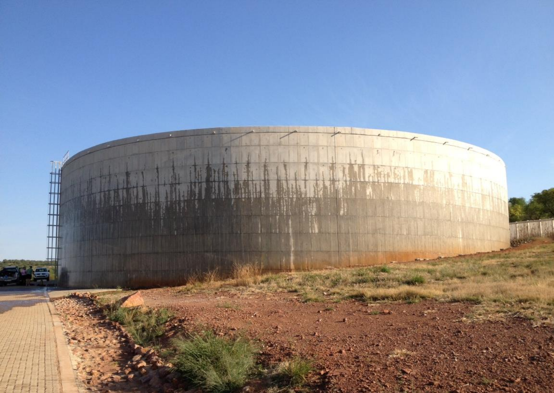
Leakage on first filling before autogenous healing.
