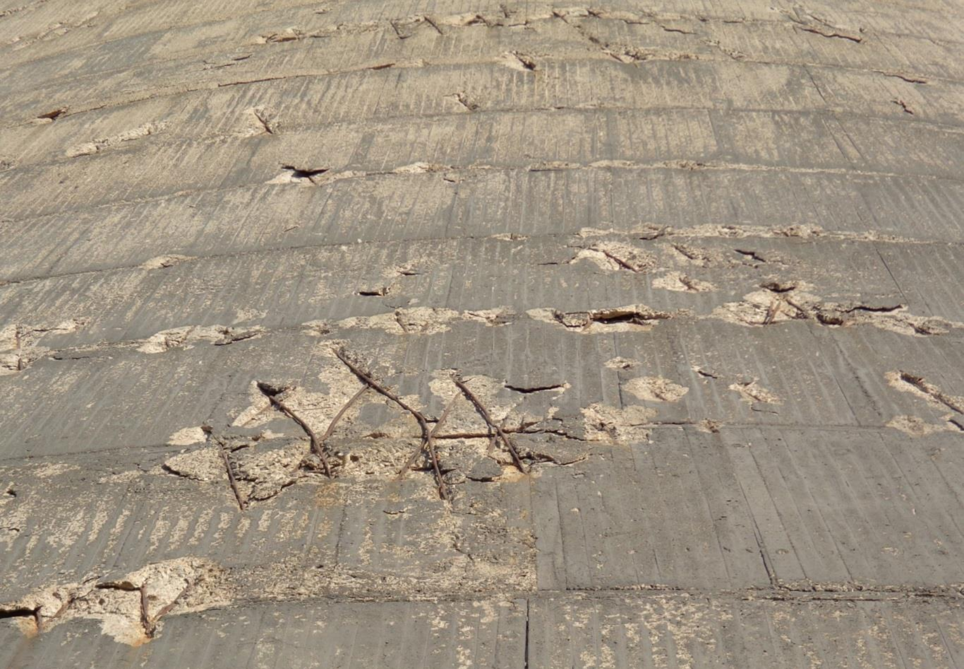
And it is at these cold-joints where rebar starts to corrode first.
