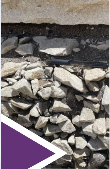
Mortar loss – exposed aggregate
